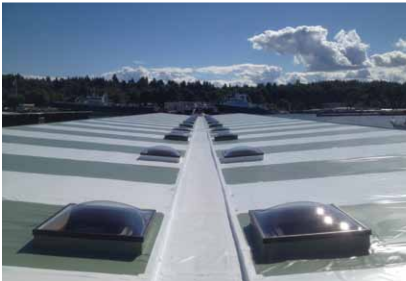
> Curb-mounted skylights were installed to replace the translucent panels in the existing metal roof. Careful framing work was required to maintain the same layout in the new roof system.
