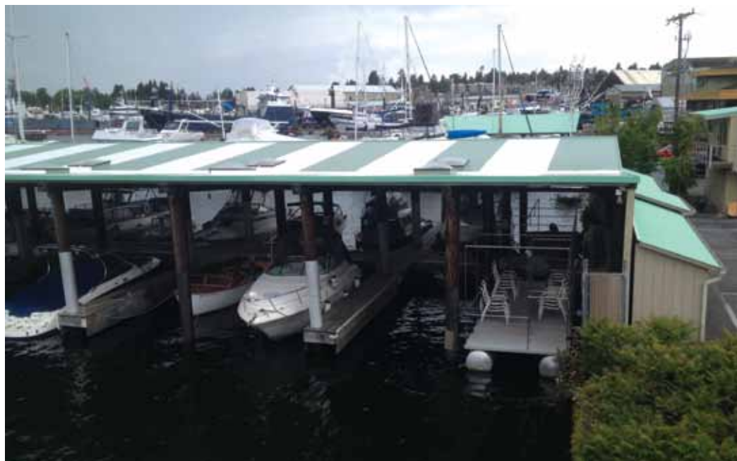
➤ Axiom Division 7 installed a FiberTite roofing system to replace the aging metal roof on the Stimson Marina in Seattle. The new roof replicates the green and white stripes of its predecessor. Photos courtesy of Axiom Division 7.
